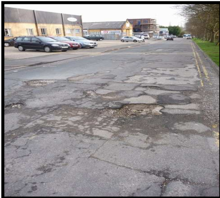
Figure 3.15.3f – Defects become more widespread.
