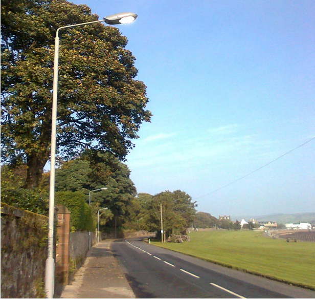
Replacement LED street lighting installed in Kilkerran Road Campbeltown. Works consisted of installing new columns, LED lanterns and new ducting and cabling.
