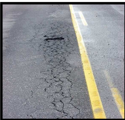
Figure 3.15.3d – Surface begins to pothole and rut.
