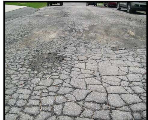
Figure 3.15.3g – Whole road surface needs replaced.
