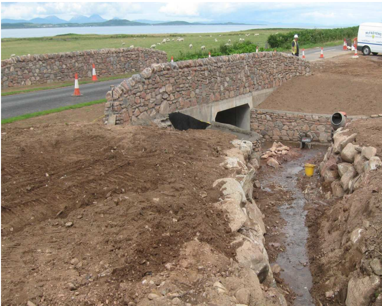
New Bridge constructed on A83 just north of Muasdale in Kintyre in July/August 2013
